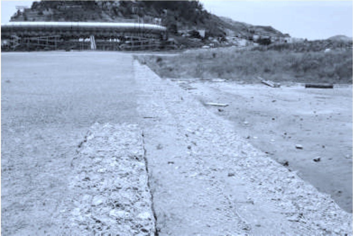
13. Promenade to the bay, Candlestick Point Cultural Park, San Francisco, by George Hargreaves Associates, 1985–93. The edge between the lawn and channel is defined by low steps constructed of gabions, wire-mesh boxes filled with stone rubble— a constructed version of the detritus found in the channels.
